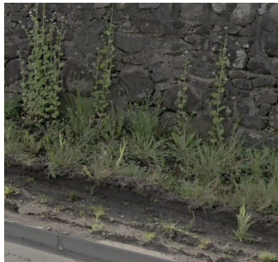
Example of minor deterioration with damaged and unmaintained verge.
