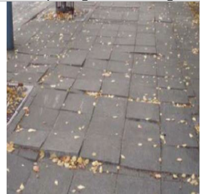
Example of major impact due to uneven and broken slabs.
