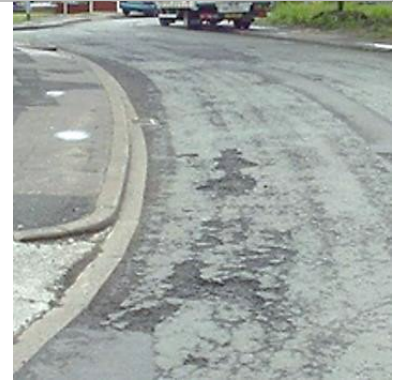
Example of major impact due to carriageway requiring resurfacing.
