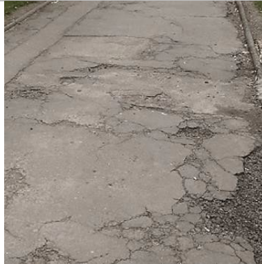
Example of major impact due to footway requiring resurfacing.
