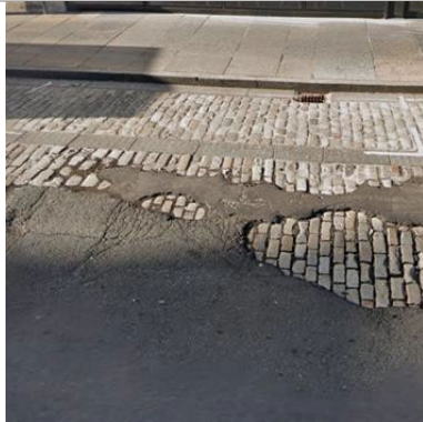
Example of major impact due to missing surface course.
