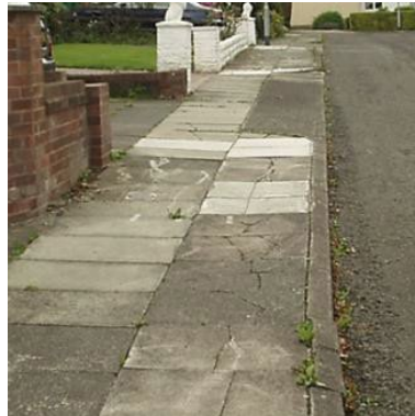
Example of minor deterioration with slabs broken and uneven.
