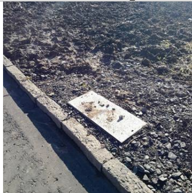
Example of major impact due to an unmade verge.
