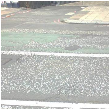
Example of minor deterioration with worn high friction, coloured and textured surfaces.
