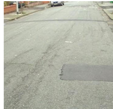
Example of minor deterioration with carriageway surface rutting.
