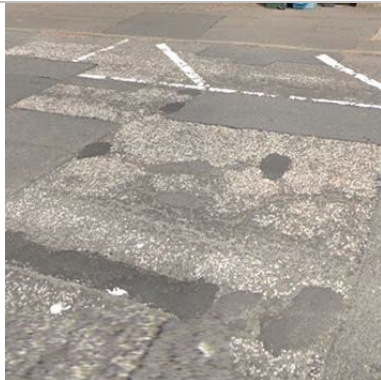
Example of major impact due to pothole repair.
