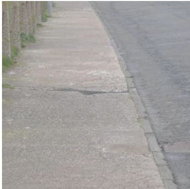
Example of minor deterioration with damaged concrete surface.
